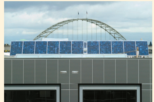
Polycrystalline roof-mounted solar panels are part of the 22.4-kilowatt system installed on Brewery Blocks Building 4.
